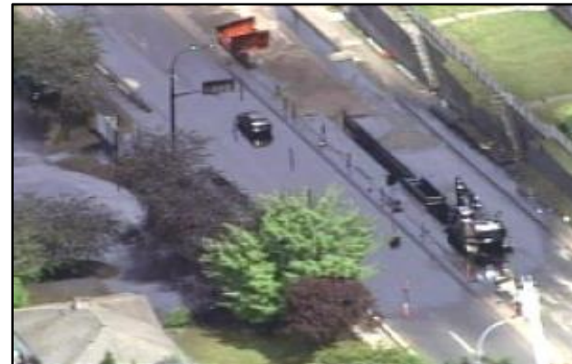
TransMountain pipeline strike (Burnaby)
